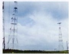
Marconi wideband wideslew centrefed dipole curtain array. R9010 similar to those to be installed in Cyprus.
