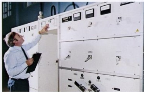
The power dividing and phase control cabinets for Radio 1 and Radio 2 at BBC Start Point.
