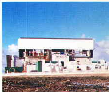
Work is proceeding at Heysham nuclear power station Stage Two. The National Nuclear Corporation is playing a major rôle in its construction for the Central Electricity Generating Board.
