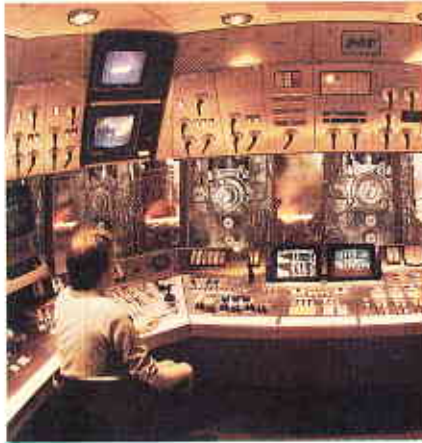
The control room of a coil plate mill in a large steel works. GEC was responsible for the complete automation system.
