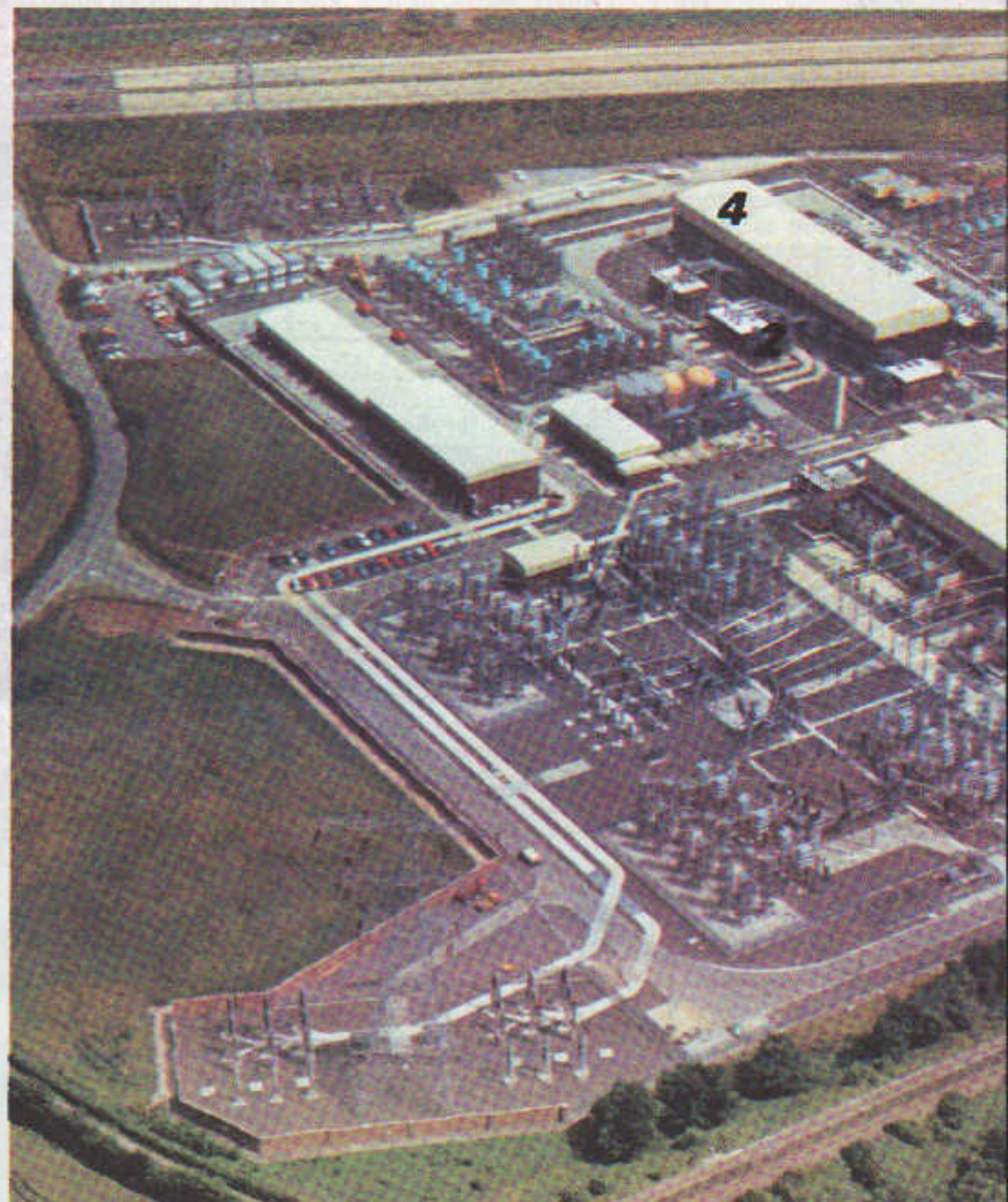
4 The converter station at Sellindge, the UK terminal of the submarine power link between Great Britain and France. See other photograph on this page.
