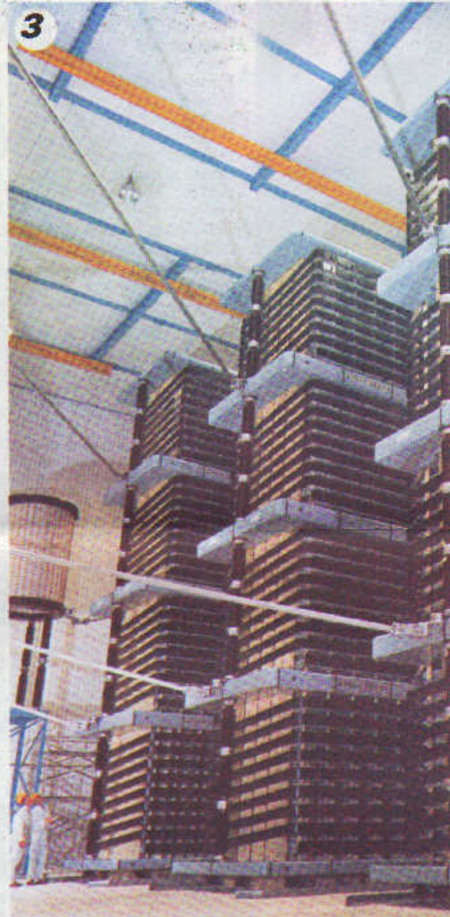
Internal view of one of the four converter valve halls at Sellindge, showing valves made by GEC Transmission and Distribution Projects.
