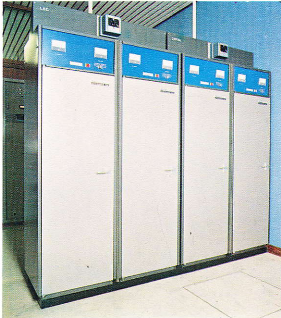
Two 1kW FM Transmitters operated by IBA for LBC and Capital Radios.
