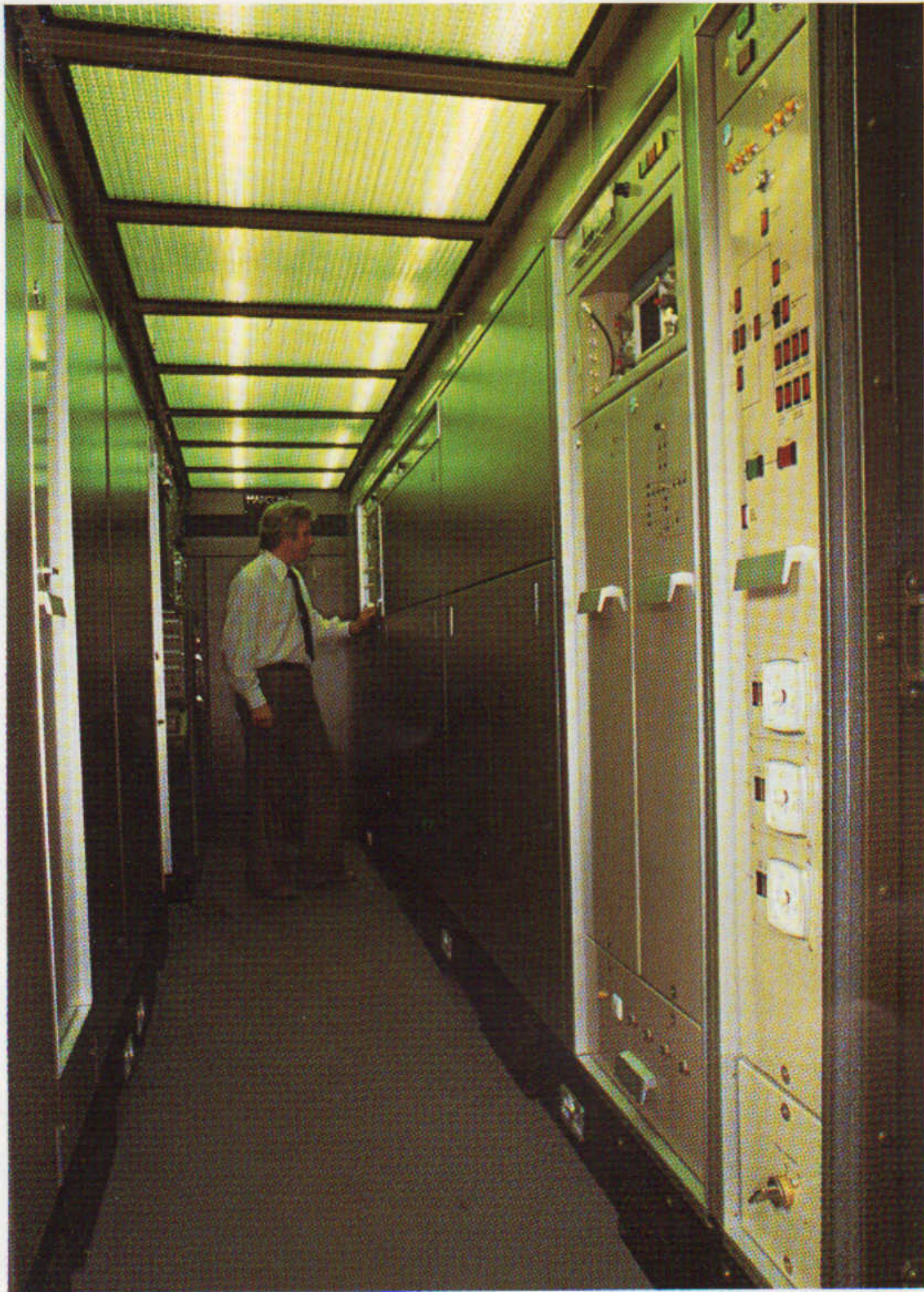
Inside the Radar Container showing the Transmitter on the right and the Signal Processing Panels and Plot-forming Cabinets opposite.
