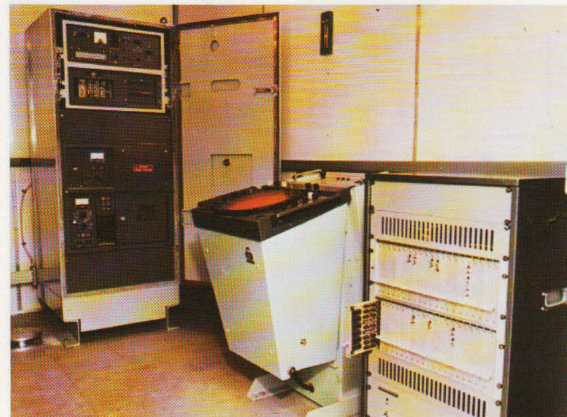
Inside cabin view of Transmitter/Receiver Cabinet, Display Unit and Signal Processor Cabinet
