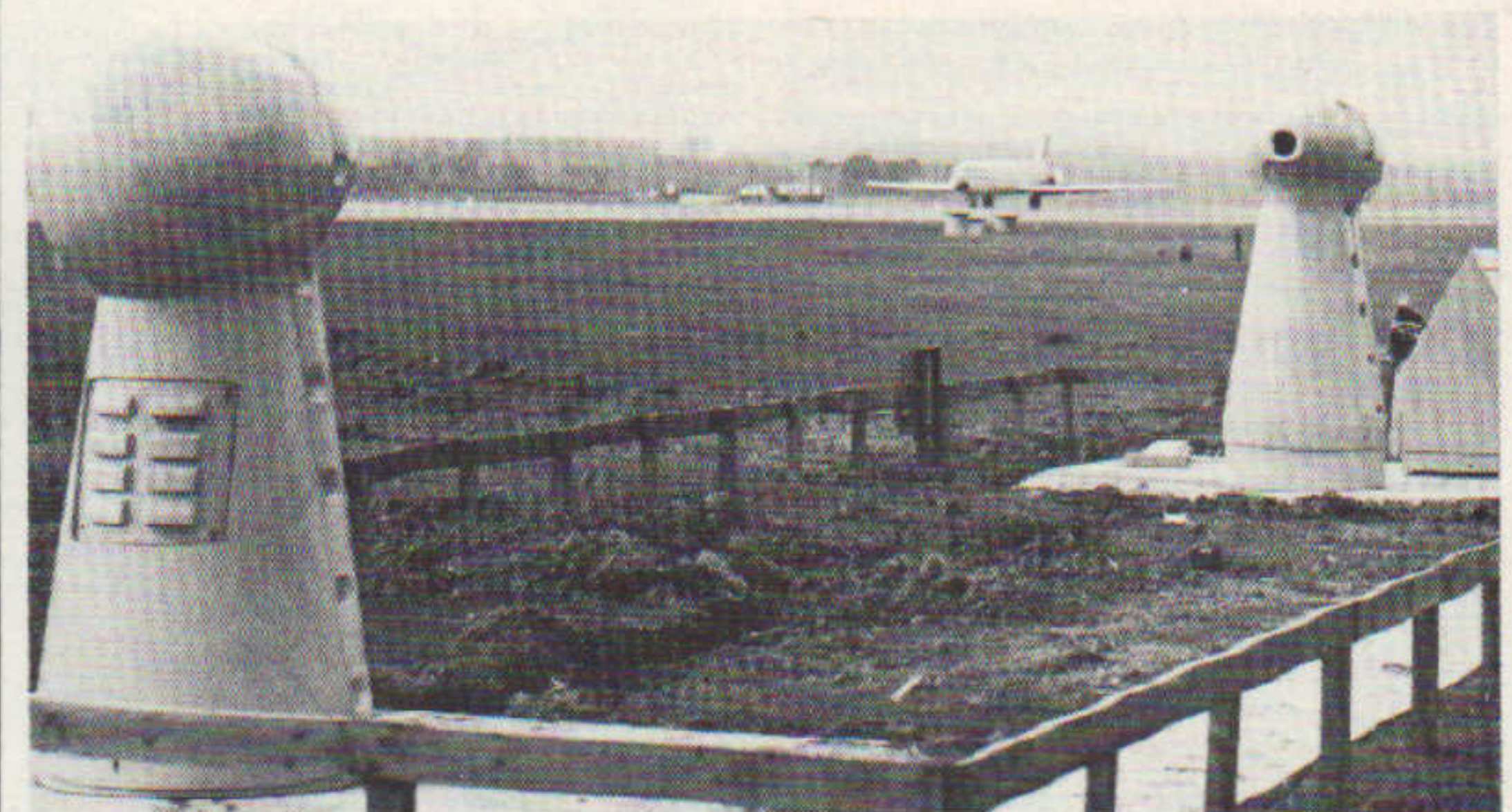
Marconi RVR installed at Gatwick Airport
