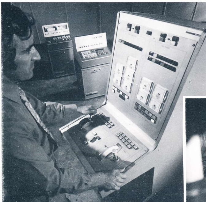
ABOVE: Jim Cooling of Loughborough University, who is a consultant to the Company, demonstrates a digital data transmission equipment for the control and surveillance of a gas turbine and three diesel generators.
