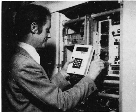
Jeff Edwards, Principal Engineer in the CMM department at New Parks, using the system's hand-held control and display unit.
