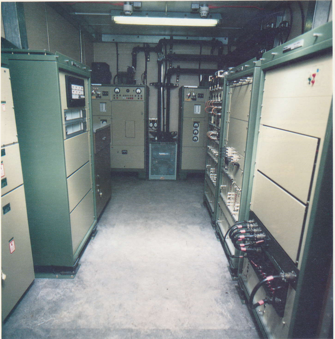
Layout of equipment in a large container
