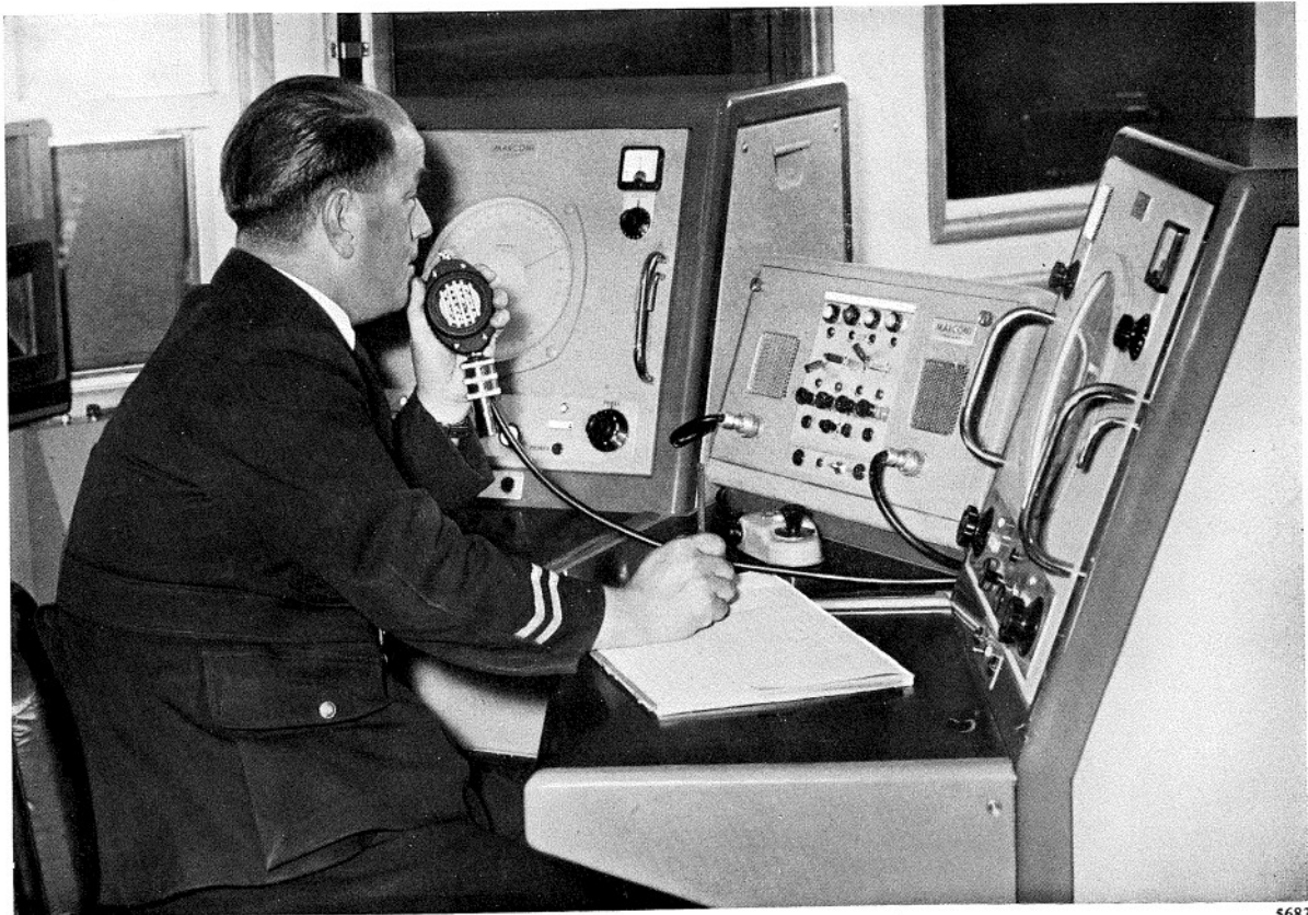
VHF Direction Finder Type AD 200 installed in the control tower at Jersey Airport.
