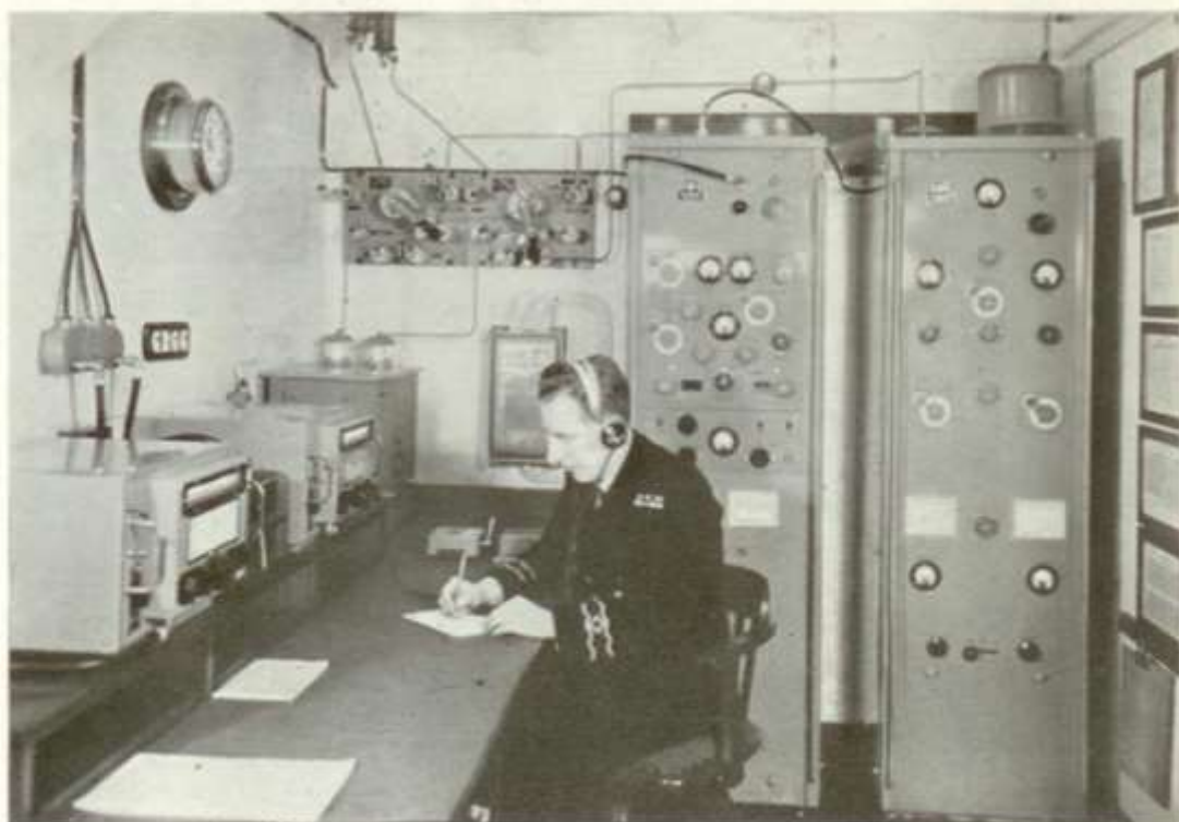
A modern radio room on board ship shows vividly the compact elegance of MARCONI marine equipment.
